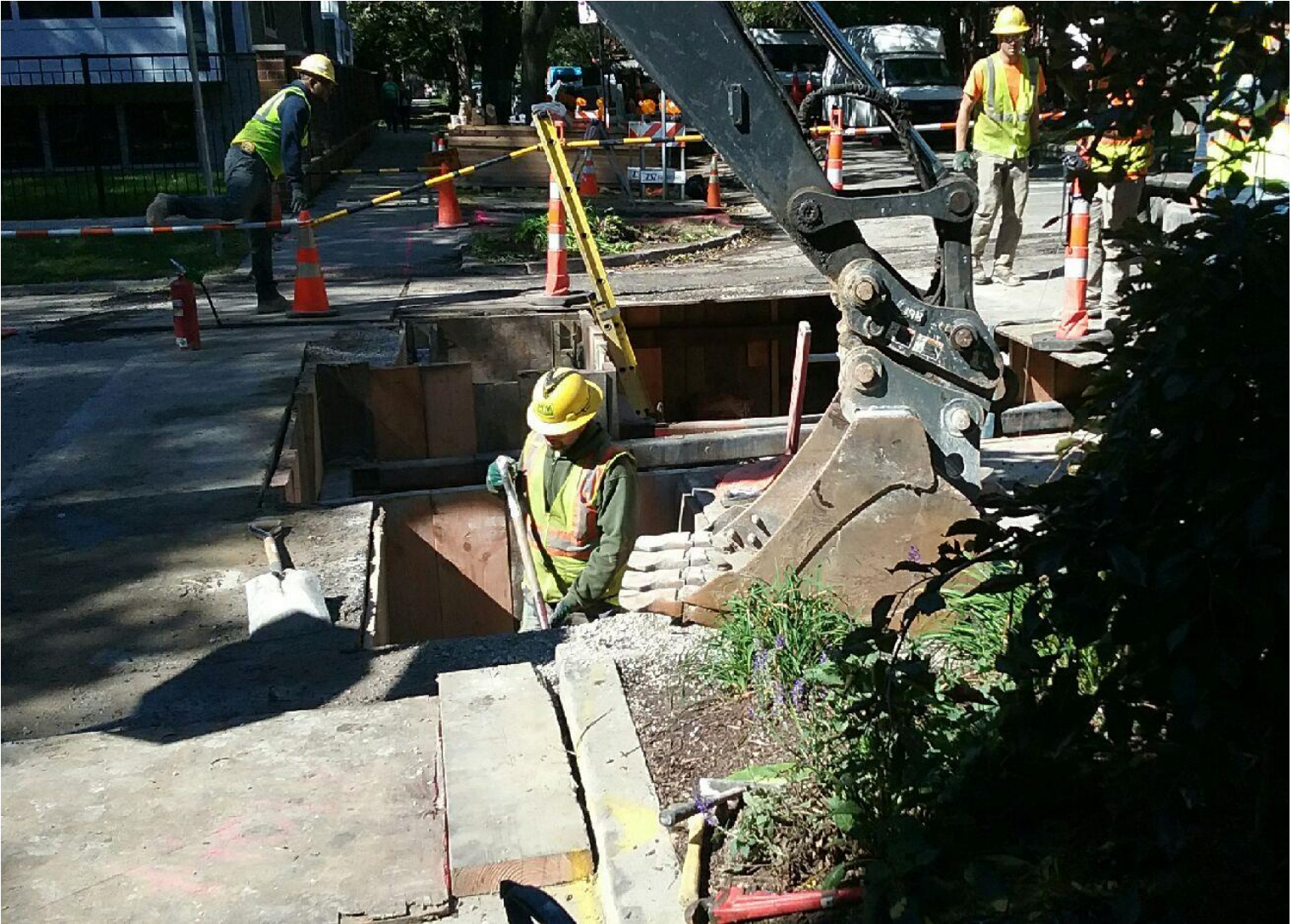
PGL North Project - Contractor completing complex shoring for a tie-in to existing gas feed.
